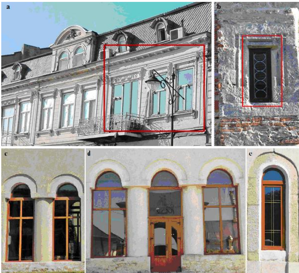
Fig. 2. Rehabilitation/modernization using thermo-insulated glass: a – Building on Tomis Boulevard, Constanta, Romania (personal photo, July 2016); b – Hadâmbu Monastery church, Schitu Hadâmbului village, Mironeasa commune, Iasi County, Romania (personal photo, July 2016); c, d and e –Hlincea Monastery church, Iasi county, Romania (personal photo, august 2016)
